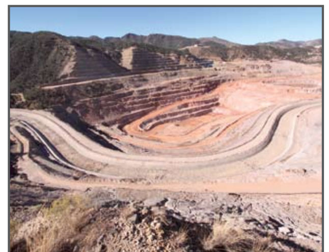
Carlota constructed the Pinto Creek Diversion to channel storm water around the mining operation.
